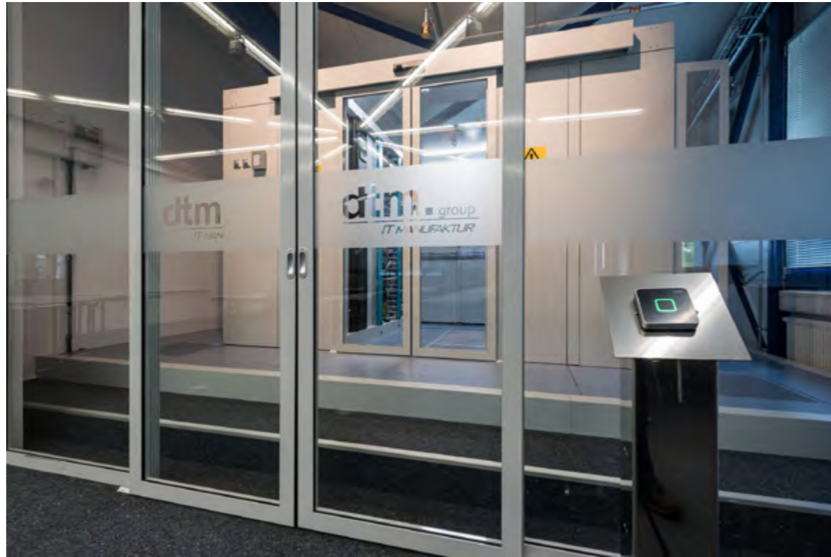
Redundant data center for training and presentation purposes
