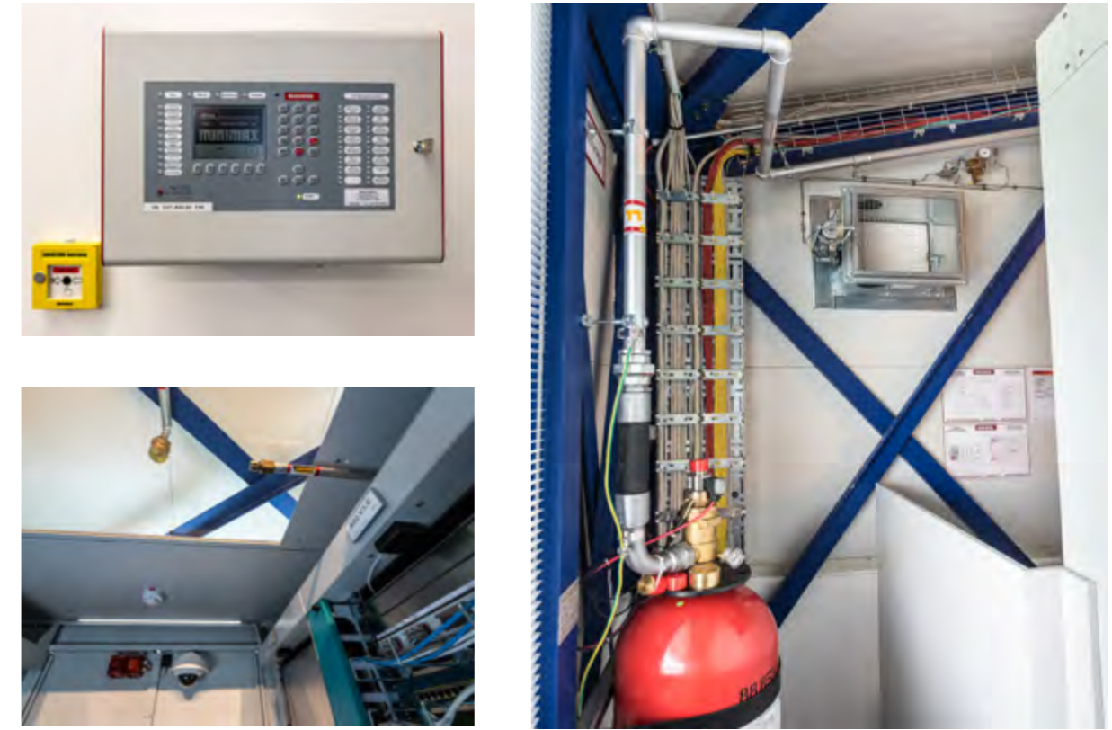
Data center in training room, safety and fire protection
